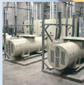
Piller central systems, SeaTac Airport, USA
