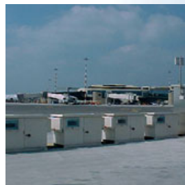
4 Apojet units, Malpensa Airport, Italy
