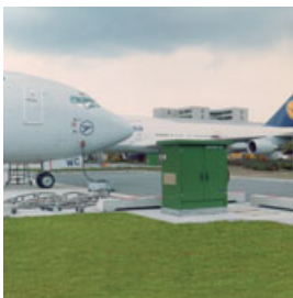
Ground power equipment, Frankfurt Airport, Germany
